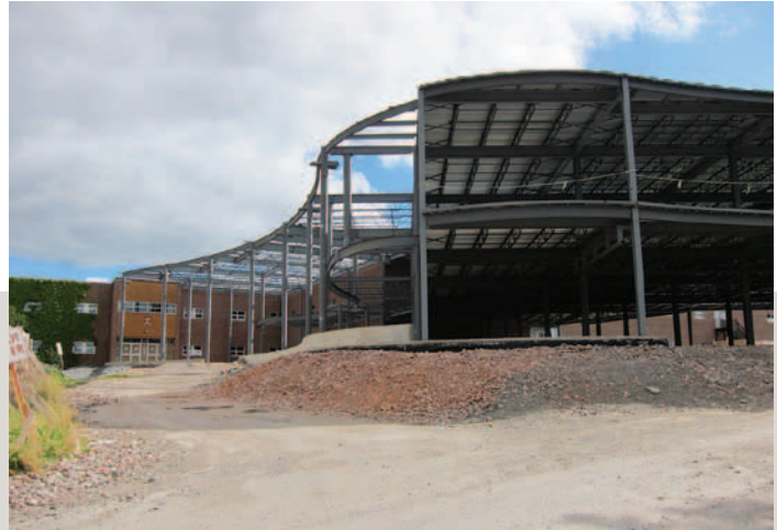
The extension will attach at the former main entrance to the Arts & Science Building
